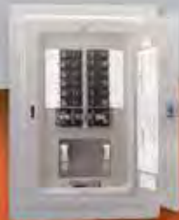
CIRCUIT PANEL UPGRADE
